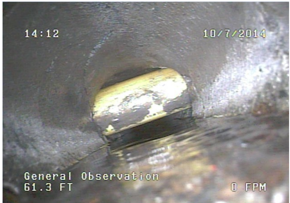
Example of a cross bore. (Courtesy Cross Bore Association)
